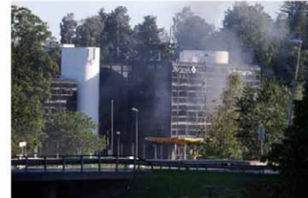
Shattered windows and damage to Office Building 65m away.
